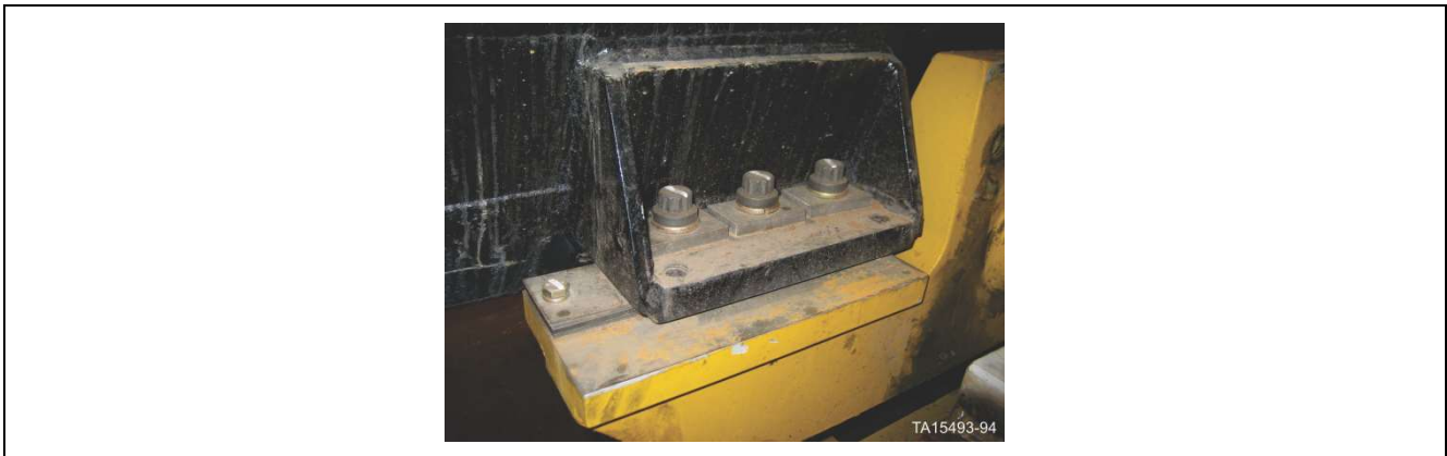
Figure 87. Generators with vertically installed bolts in mounting feet
