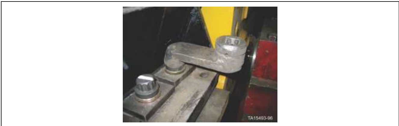
Figure 192. Offset adapter may be required to torque the bolts on the generator
