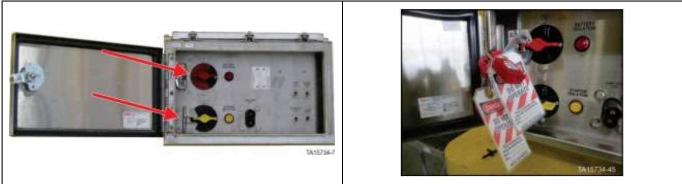
Battery Isolation Box – Battery isolation switch in OFF position with locks in place
