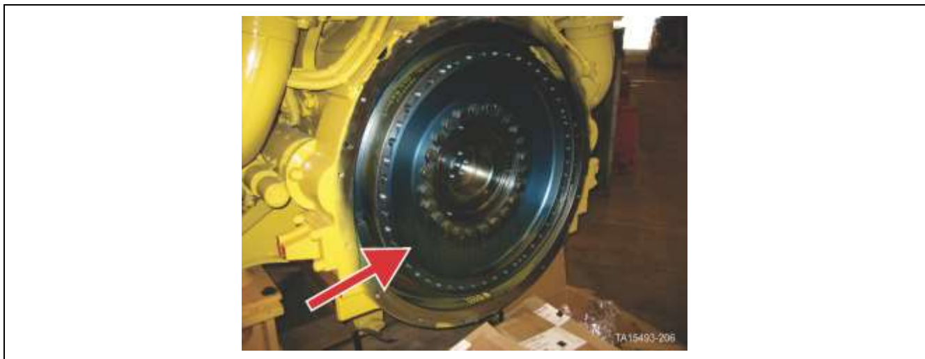
Figure 267. Measurement of Radial Runout of Engine Flywheel - Tier 2 DD/MTU
