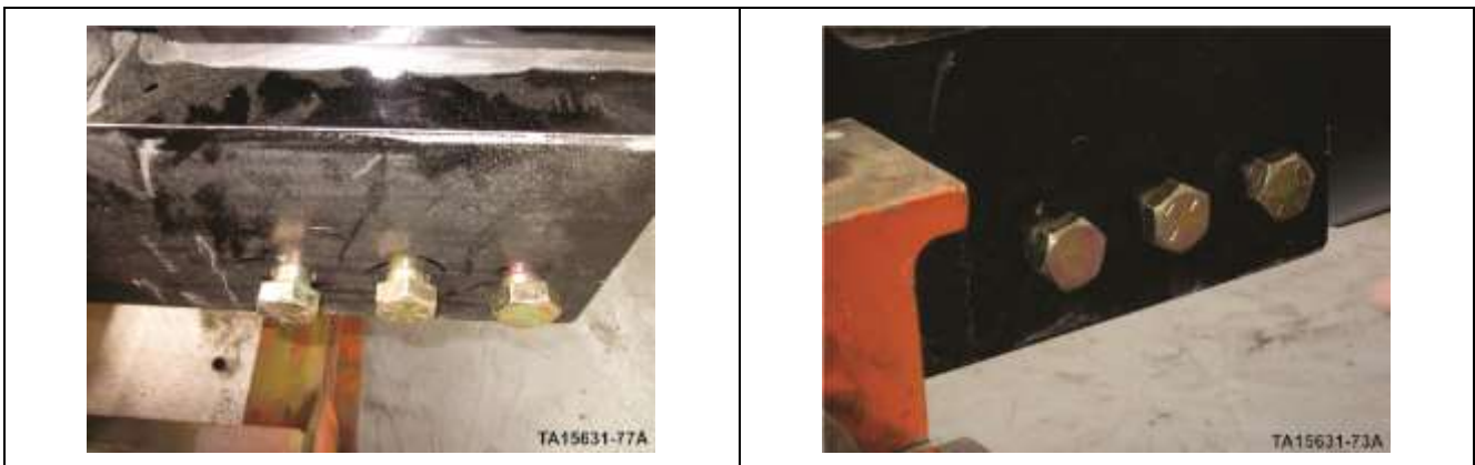
Figure 88. Generators with horizontally installed bolts in mounting feet
