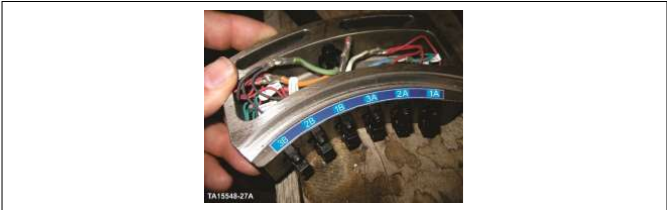
Figure 14. SR generator RPT assembly
